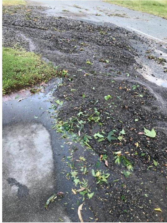
Gravel washed onto Gladstone Street, Hall
