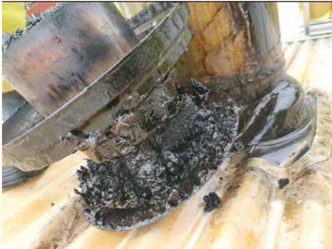
Carbon build-up in a flue – a chimney fire in the making
