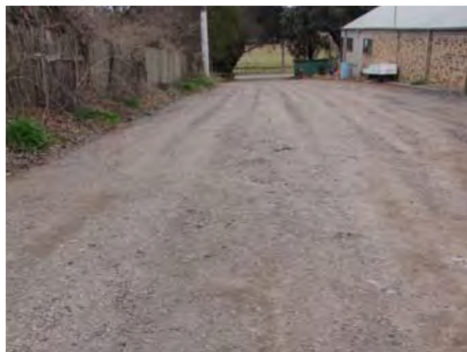
Bootmakers Lane gets the attention it deserves. New millings, grading and drains cleared.
