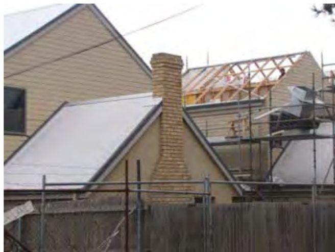
Victoria Square Development news flash! Work has begun to rectify the the deviations from the development application.
